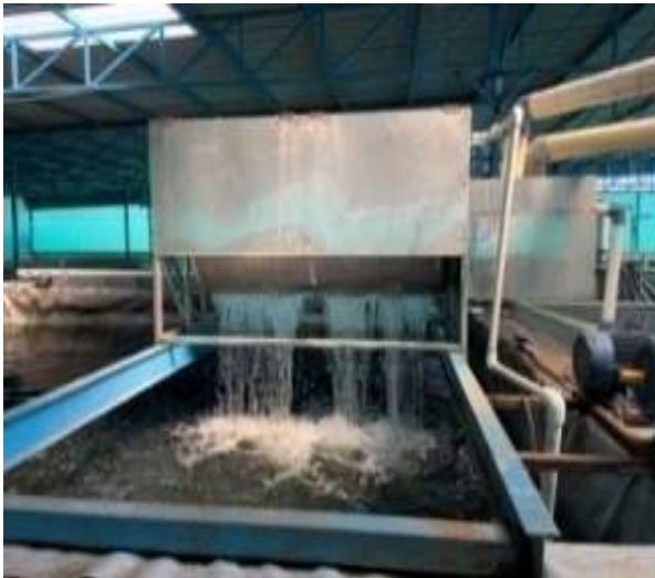
Figure 1: Representation of malfunctioning of the working drum filter
